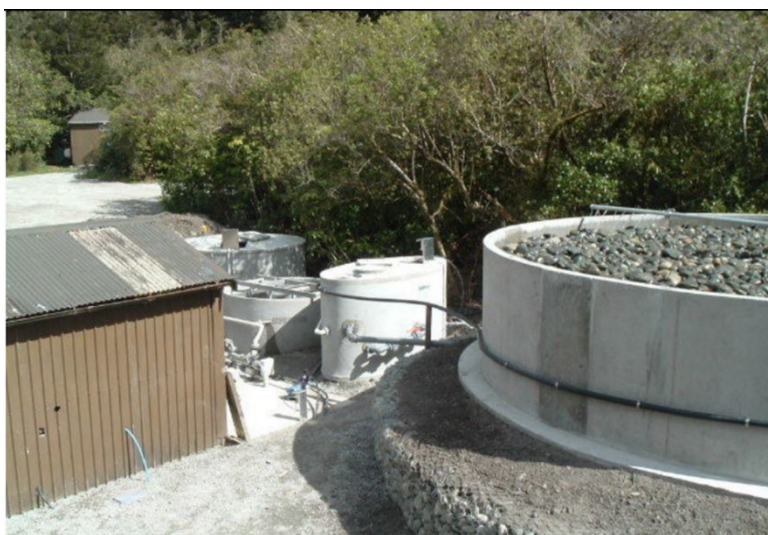
Figure 4: Wastewater treatment plant at Deep Cove
